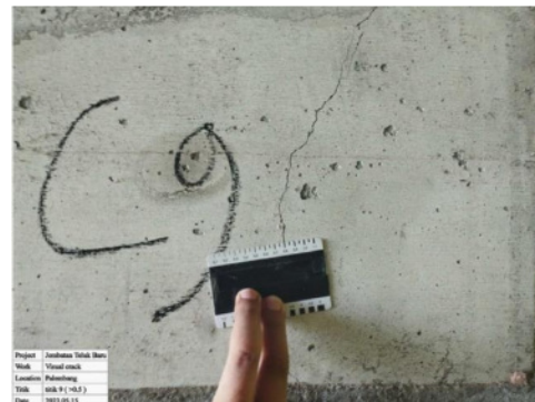
(b) Crack on concrete box girder web
